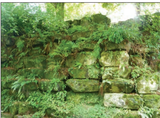
Figure 13. Supportive Rockwork in Pittencrieff Glen Close to the Double Bridge. Photograph author's own.
