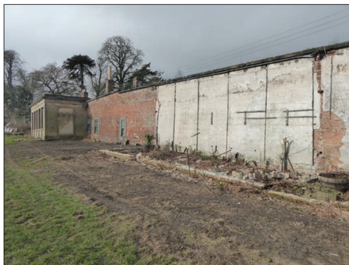
Forcett Hall. South Facing Wall with Orangery/Pavilion and the area where the Richardson Glasshouse had stood
